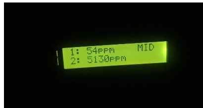
Figure 8 Gas Leakage System Results
